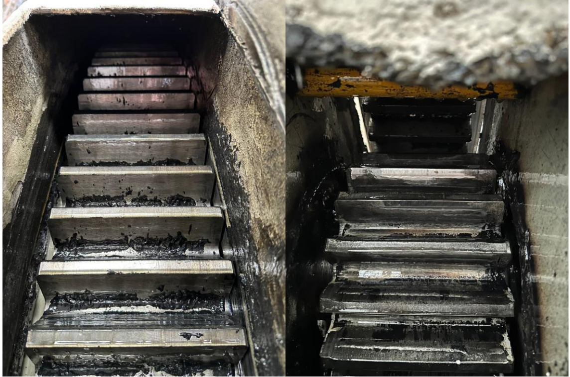
Figure 10. Photographs of the spalled gears and Lubrication problem
